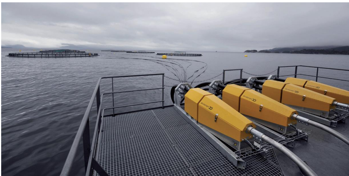
Figure 16: Example of an automated AKVA Feeding System
